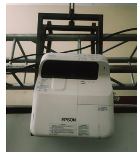
Figure 7. Front View of the Floor Projector After Final Installation.
